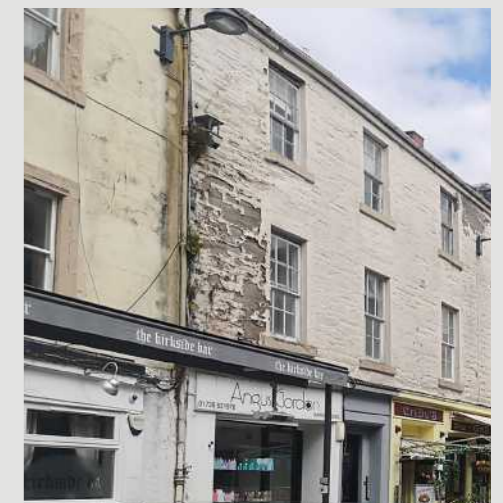
Example of building maintenance issues
